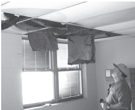
Mike Davis, assistant vice president for administration, inspects post-Gustav ceiling damage in South Babington Hall.
