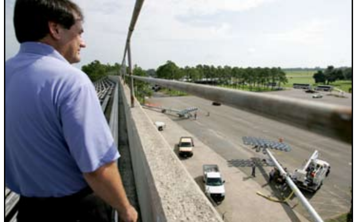
Brian Clausen, director of environmental health and safety, observes as work crews prepare to lift the new lights at John L. Guidry Stadium.
